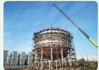
The pictures provided by visualisation system - construction site of LNG storage facilities in city-gate station
