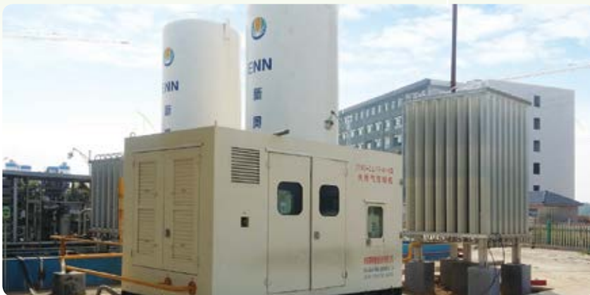
LNG refuelling station equipped with residual gas recovery equipment
